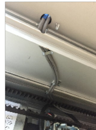
Example of sensor cable routing on backside of cover into header.
